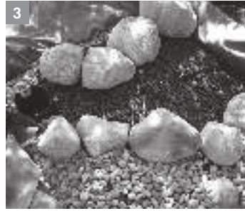
Step 3 – Fill in gaps with gravel and set boulder edges. Fold remaining liner over matrix and cover with rocks and dirt
